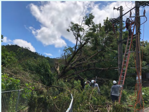
Extreme weather events such as typhoons pose significant risks to the operation and structure of overhead lines in Hong Kong.
