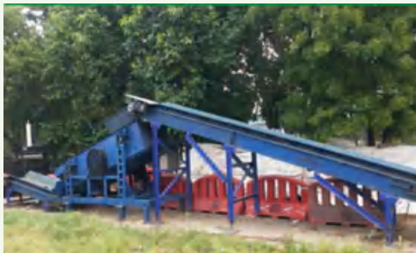
Vibro-Feeder used at the Material Recovery Facility at Jhajjar Power Station.
